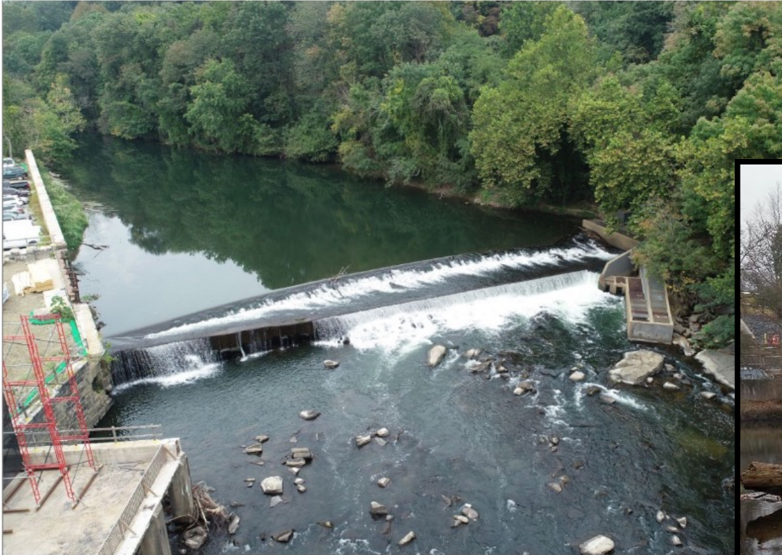
Photo 1. Aerial View of Dam 4 from Drone Showing Void on Left Side, Dated 9/2
