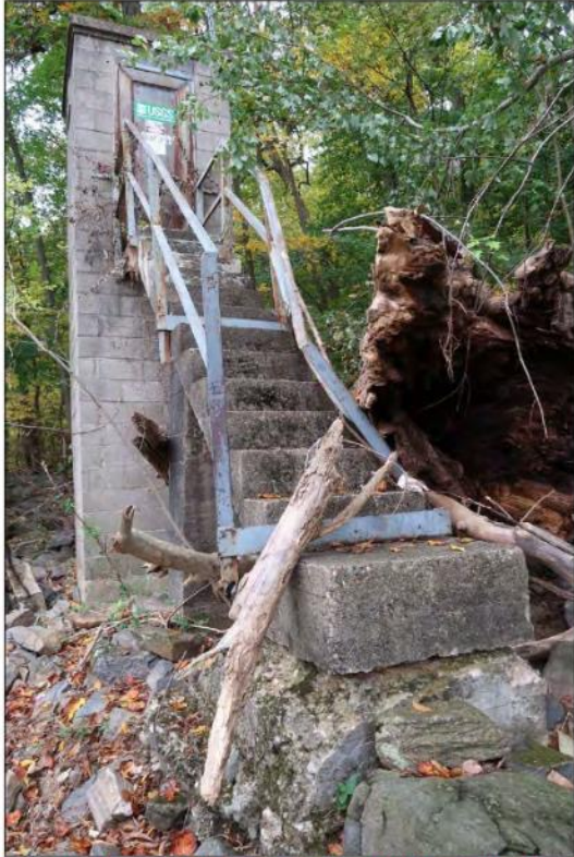
Figure 132. View of the USGS Water Monitoring Station Gage House, looking east, 2021. (Center for Historic Architecture and Design)
