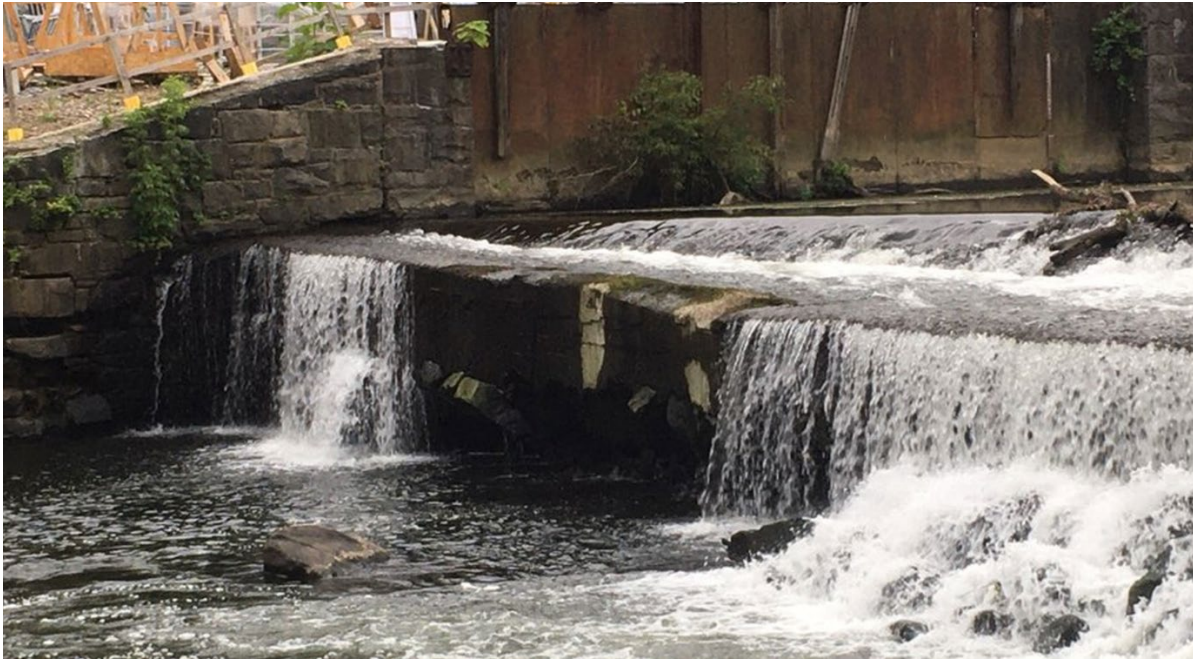
Photo 2. Downstream Face of Dam 4 Showing Void, Dated 8/04/2020
