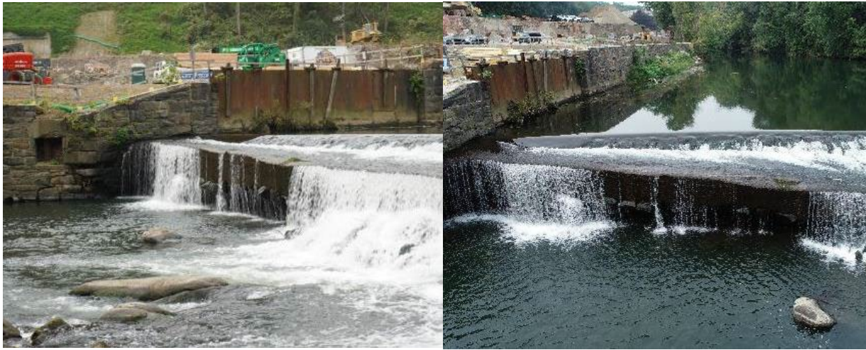
Figure 2. Dam 4 Potentially Undermined Section, Looking Upstream at the Right Abutment (left photo) and area of instability (right photo)
