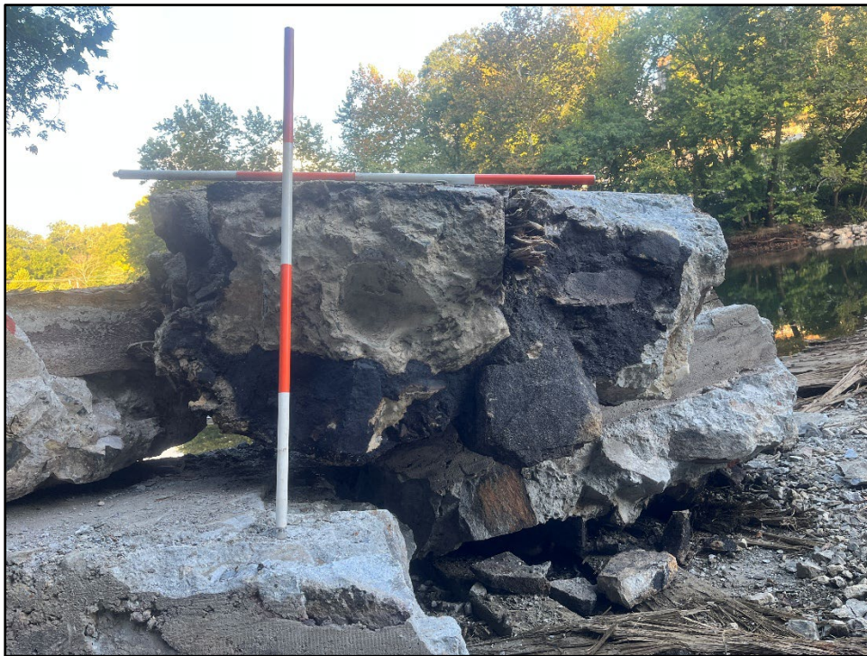
Plate 4.8: View of the cross section of a portion of the concrete top removed from the dam. Photo view: N/A; Photographer: Jonathan E. Dernbach; Date: August 2, 2025.
