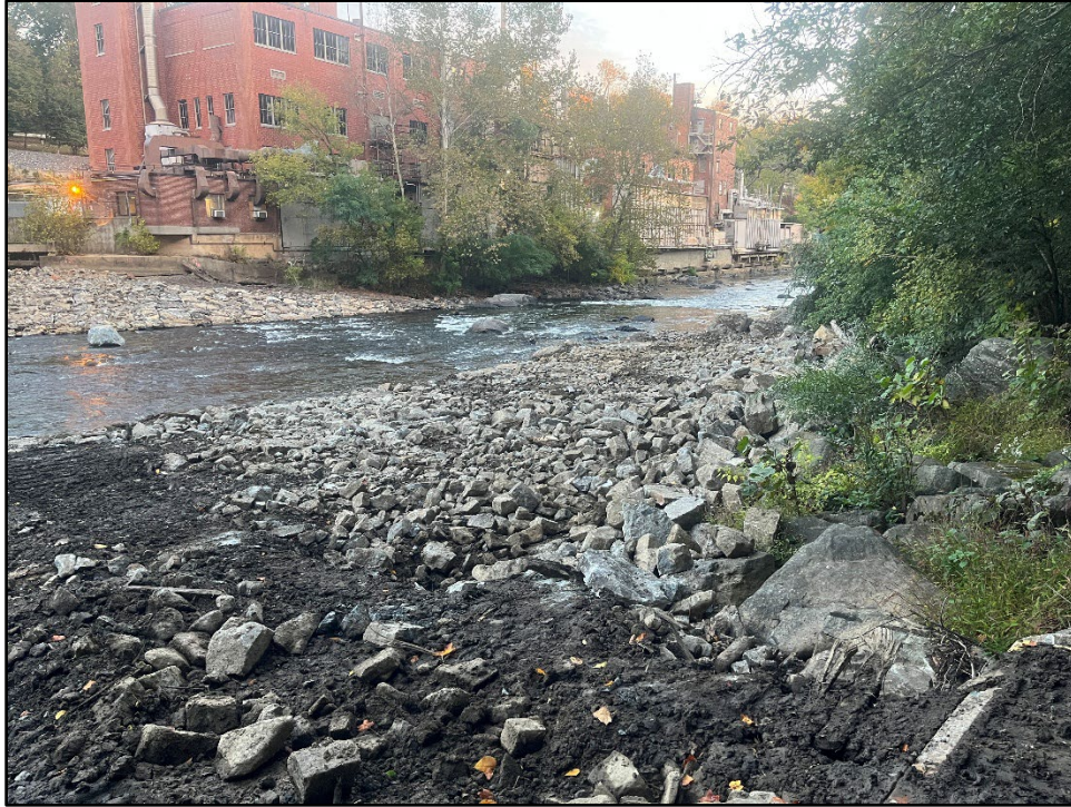
Plate 4.27: View of the stone and concrete debris placed along the southern side of Brandywine Creek during the removal process Photo view: Northeast; Photographer: Jonathan E. Dernbach; Date: October 15, 2025.
