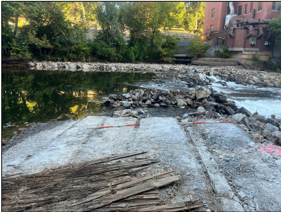
Plate 4.16: View of the upper concrete face of the dam at 50 percent breach showing the concrete strips and upright, milled boards. Photo view: Northwest; Photographer: Jonathan E. Dernbach; Date: August 2, 2025.
