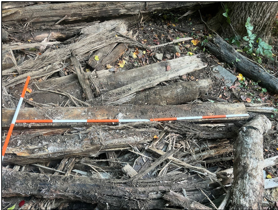
Plate 4.6: View of the end of an intact milled board removed from the dam structure. Photo view: N/A; Photographer: Jonathan E. Dernbach; Date: October 15, 2025.
