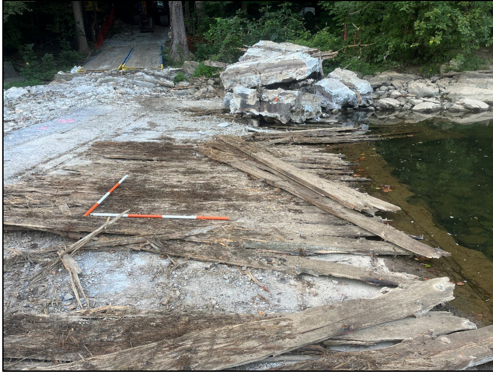
Plate 4.17: View of top of the dam at its southern abument showing wooden planking covering the upstream, sloped portion of the dam. Photo view: South; Photographer: Jonathan E. Dernbach; Date: August 2, 2025.
