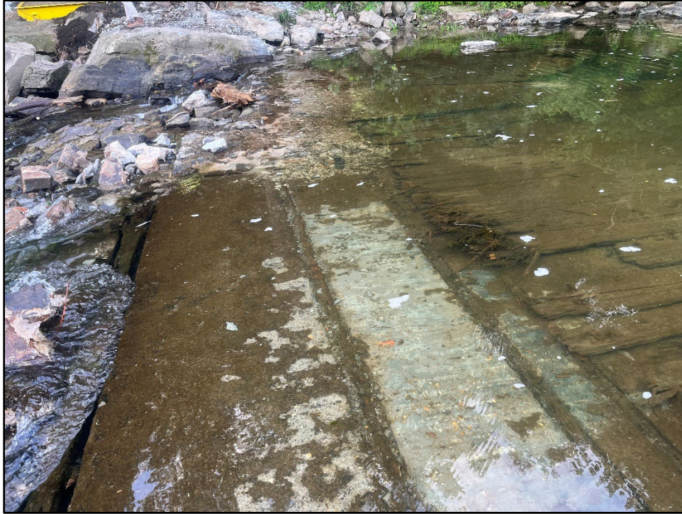
Plate 4.3: View of the southern abutment of Brandywine Dam 6 showing concrete strips with milled timbers and wooden planks on the upstream side of the dam. Photo view: Southeast; Photographer: Jonathan E. Dernbach; Date: July 23, 2025.
