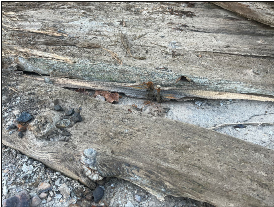
Plate 4.20: View of planks and fasteners on the upstream portion of the dam.
