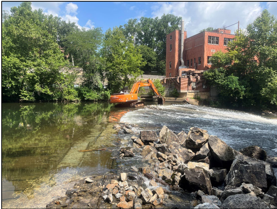
Plate 4.4: View of the removal work in progress at Brandywine Dam 6. Photo view: Northwest; Photographer: Jonathan E. Dernbach; Date: July 23, 2025.
