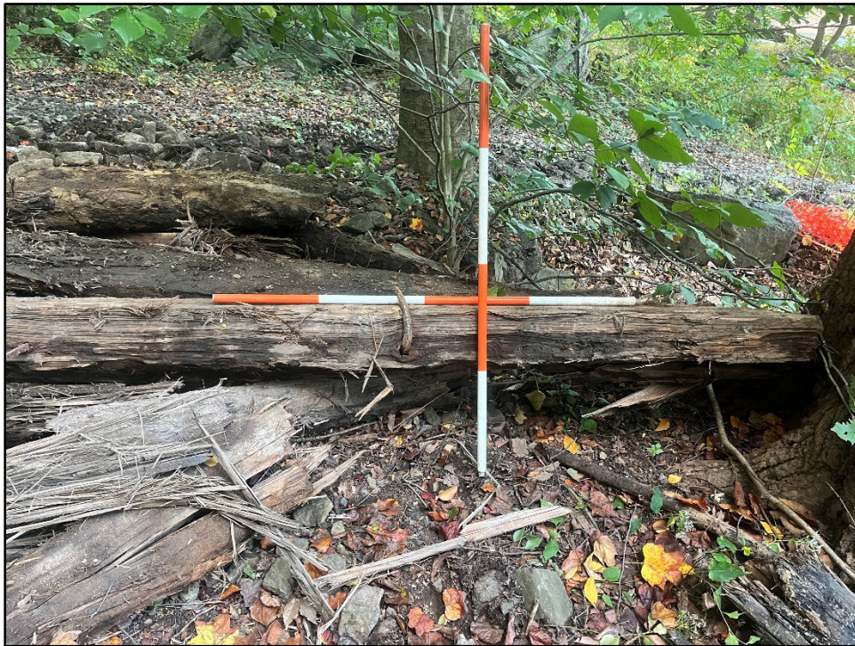
Plate 4.22: View of a large, square timber with a 2-foot ferrous metal spike removed from the lower portion of the dam structure near 100 percent breach. Photo view: N/A; Photographer: Jonathan E. Dernbach; Date: October 15, 2025.
