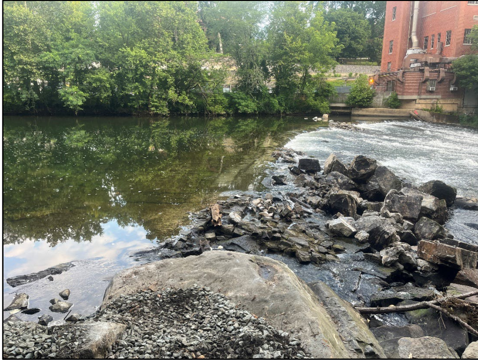
Plate 4.1: Overview of Brandywine Dam 6 from its southern abutment after the initial breach.
