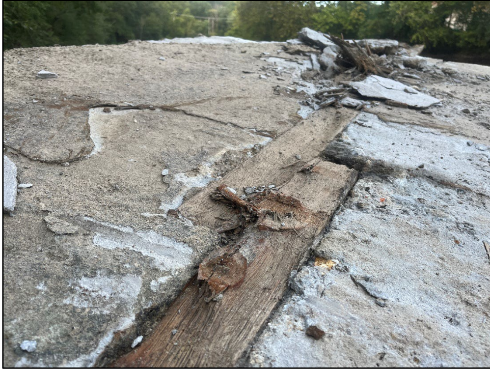
Plate 4.7: View of overlapped, milled boards on the upper surface of the concrete top . Photo view: N/A; Photographer: Jonathan E. Dernbach; Date: August 2, 2025.
