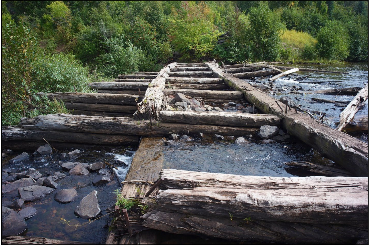
Figure 4.7: A photograph of a typical timber crib dam in Redridge, Michigan that is similar to observations of the underlying structure of Brandywine Dam 6. Note the large ferrous metal spikes at joints. (Rexp2 2013).
