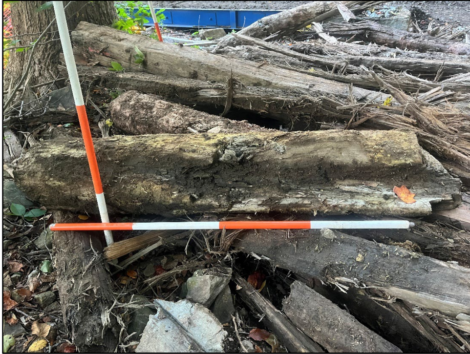
Plate 4.25: View of a circular log removed from the lower portion of the dam structure near 100 percent breach.
