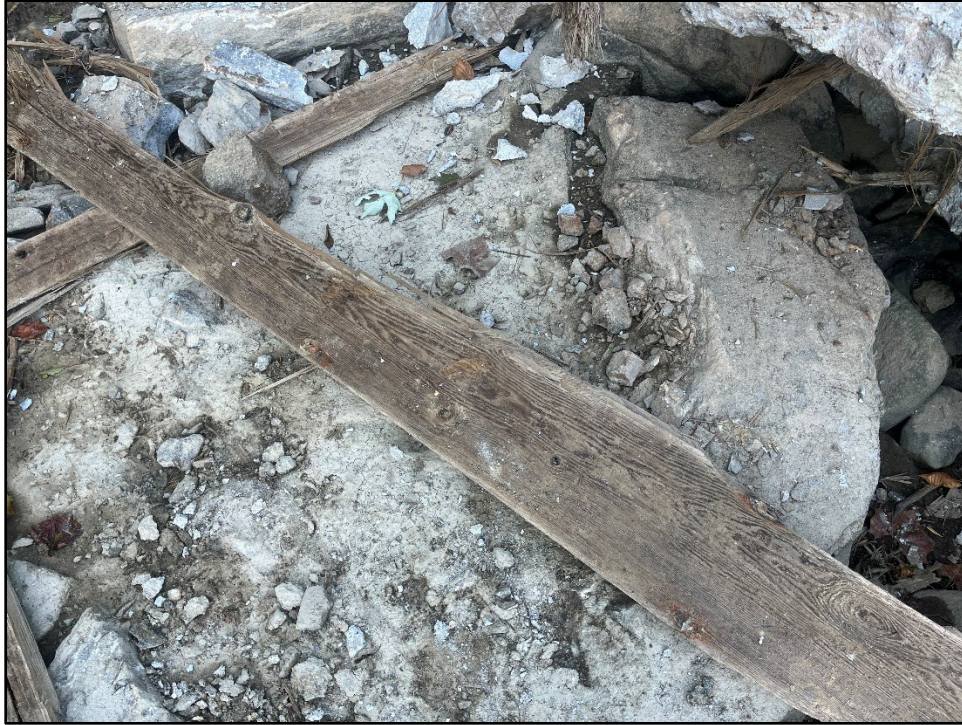
Plate 4.19: View of the upper surface of a wooden plank removed from the downstream, sloped portion of the dam.
