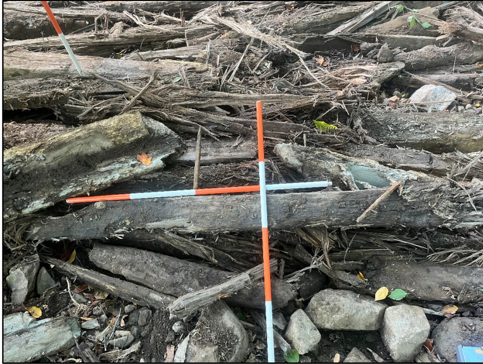
Plate 4.23: View of a large, square timber with 2-foot ferrous metal spikes removed from the lower portion of the dam structure near 100 percent breach. Photo view: N/A; Photographer: Jonathan E. Dernbach; Date: October 15, 2025.
