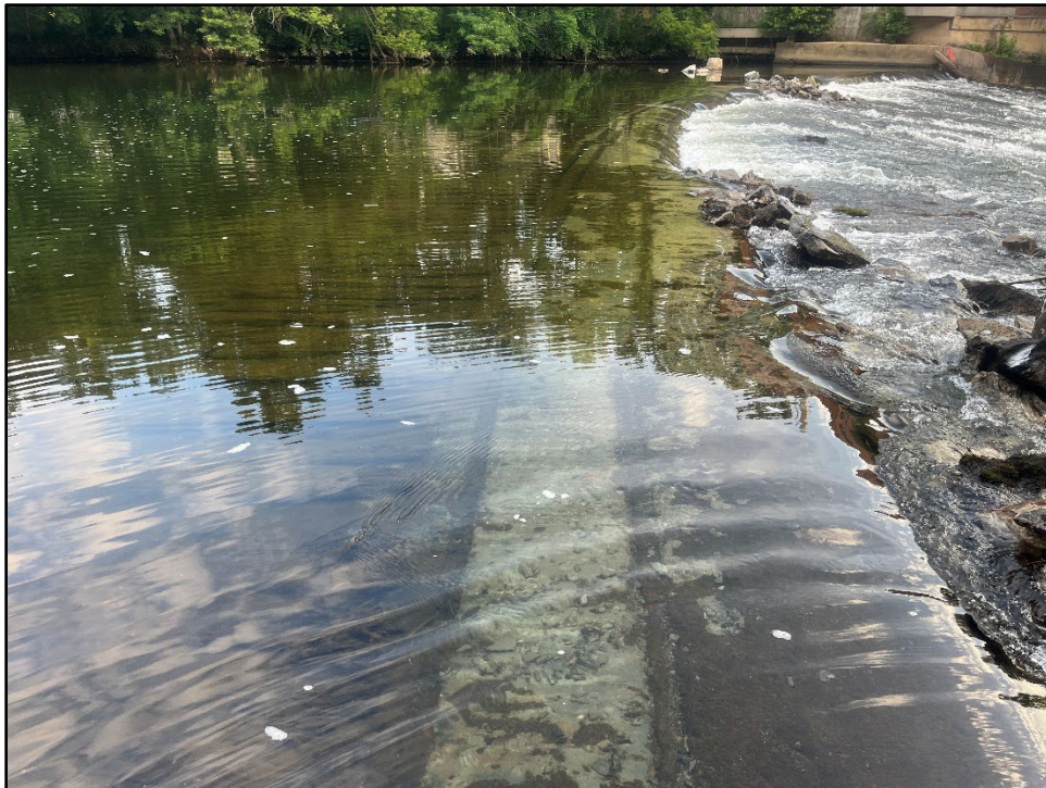
Plate 4.2: Closeup view of the top of Brandywine Dam 6 following the initial breach.
