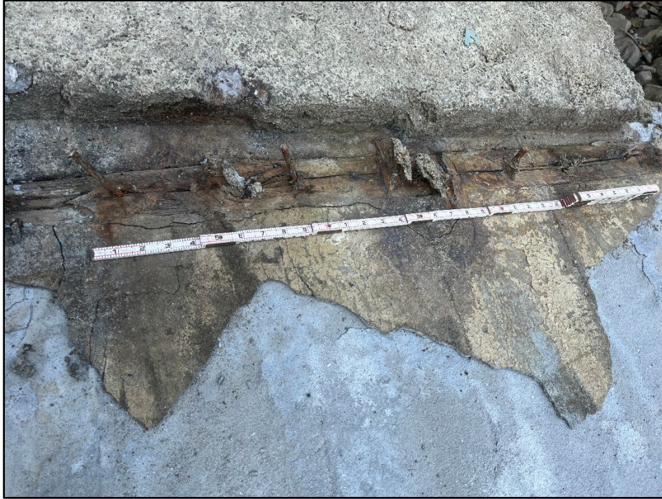
Plate 4.21: View of the upper surface of a portion of the concrete dam topvshowing fasteners used to attach the wooden planking to the upright, milled boards on the upstream side of the dam. Photo view: N/A; Photographer: Jonathan E. Dernbach; Date: August 2, 2025.
