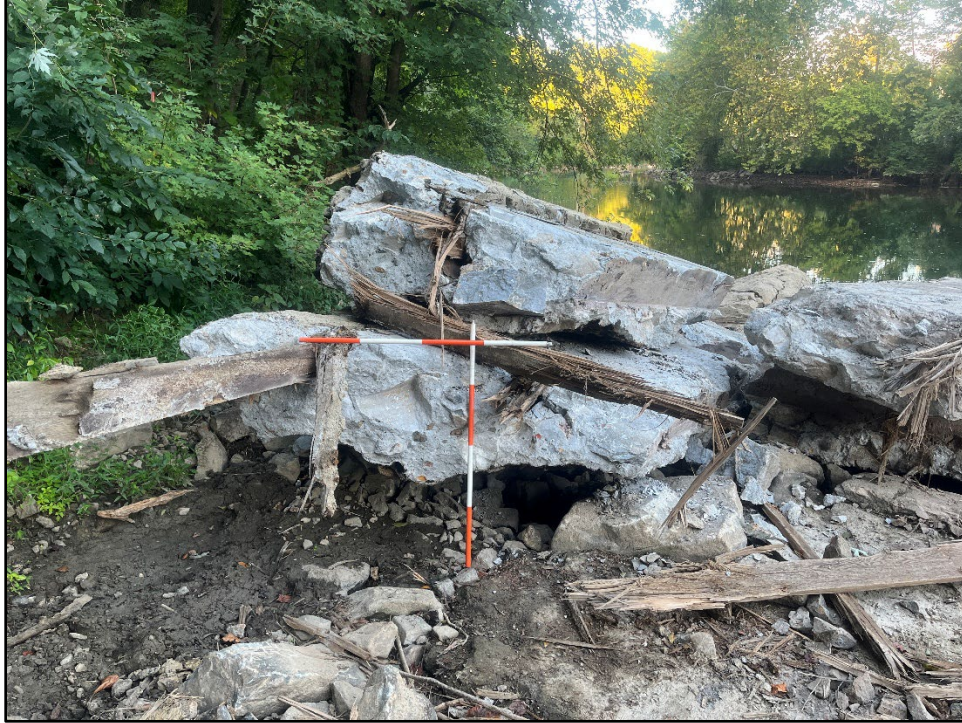
Plate 4.9: View of the cross section of a portion of the concrete top removed from the dam showing milled boards.
