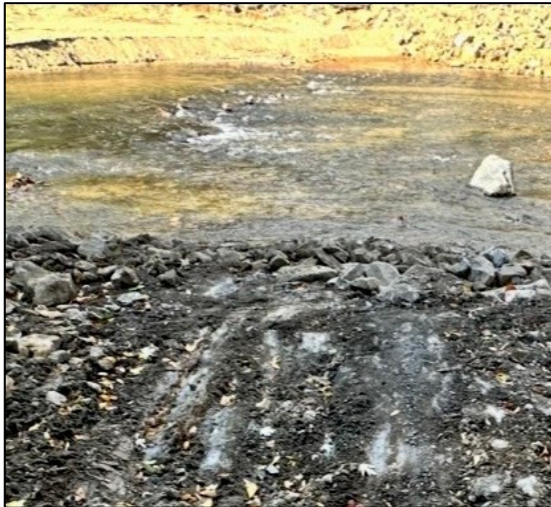
Plate 4.26: View of the remaining portion of the dam at the southern abutment following the completion of excavation/removal.
